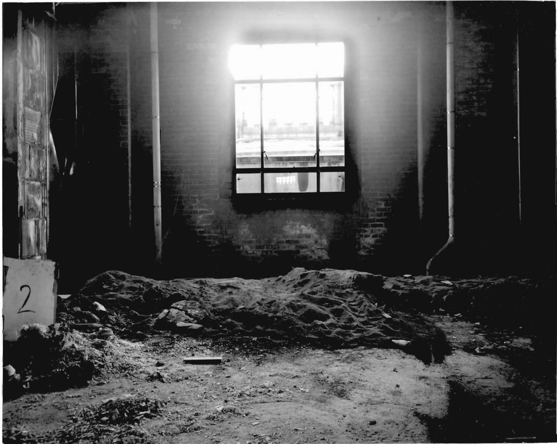
2. VIEW OF WINDOW ON EAST SIDE OF 20TH FLOOR SHOWING POSITION OF BALUSTRADE OUTSIDE OF WINDOW
