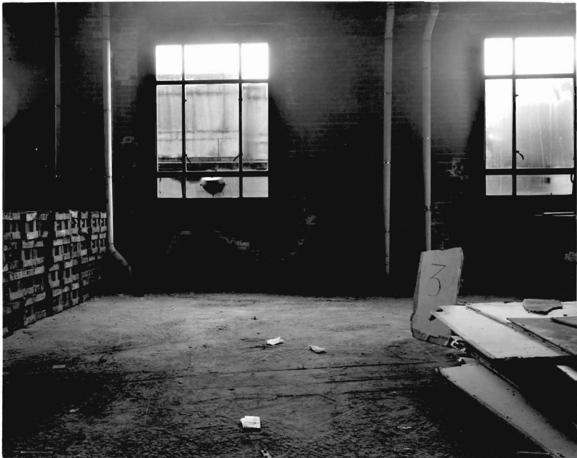
3. VIEW OF WINDOW ON NORTH SIDE OF 20TH FLOOR SHOWING POSITION OF BALUSTRADE OUTSIDE OF WINDOW
