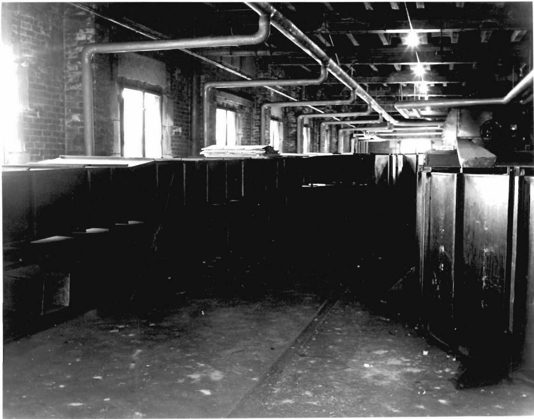
8. 24TH FLOOR (PIPE & DUCT FLOOR) SUN LIFE BUILDING, MONTREAL.
