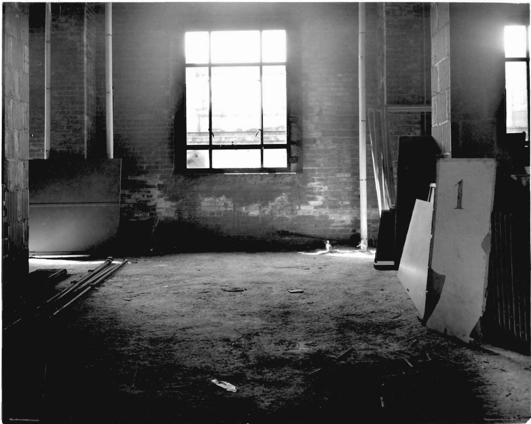
1. VIEW OF WINDOW ON WEST SIDE OF 20TH FLOOR SHOWING POSITION OF BALUSTRADE OUTSIDE OF WINDOW
