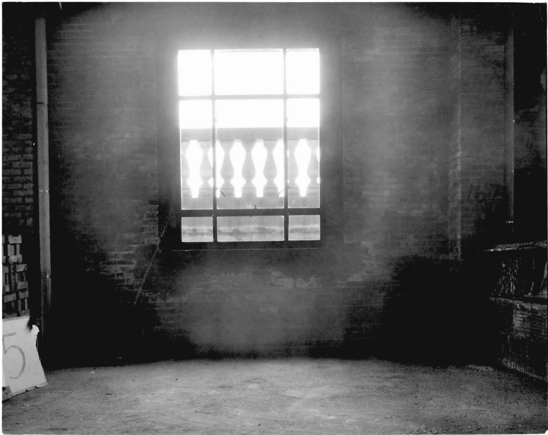
8. VIEW OF WINDOW ON EAST SIDE OF 23RD FLOOR SHOWING POSITION OF BALUSTRADE OUTSIDE OF WINDOW
