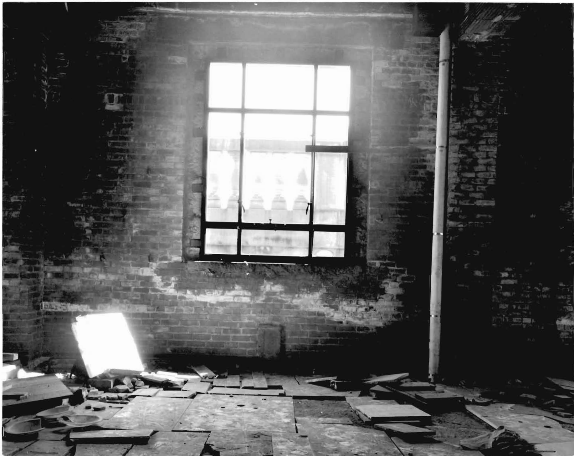
7. VIEW OF WINDOW ON SOUTH SIDE OF 23RD FLOOR SHOWING POSITION OF BALUSTRADE OUTSIDE OF WINDOW
